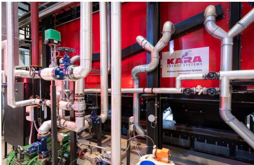
Biomassacentrale in Lochem.
