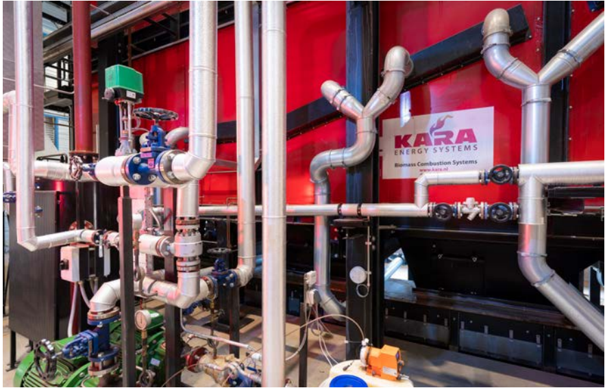
Biomassacentrale in Lochem.
