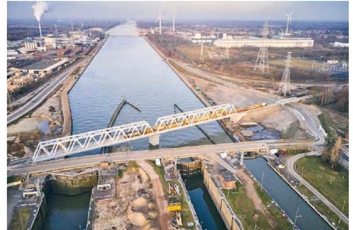
Construction works on the railway bridge crossing the Albert Canal near Genk.
